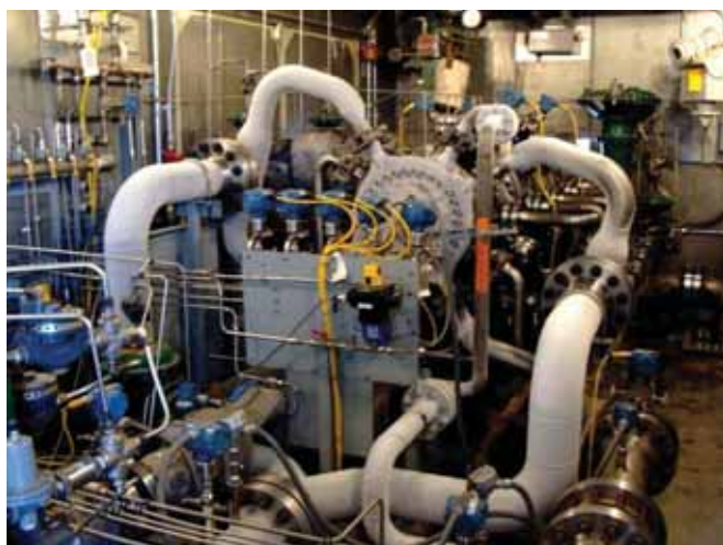
The combustor carefully reacts natural gas with oxygen
