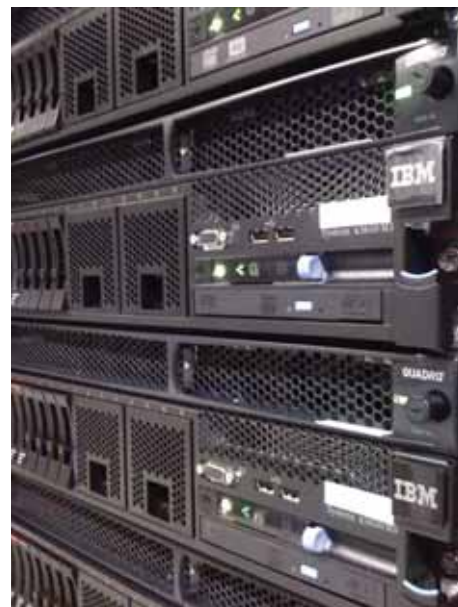
Santos' Turbo VNC servers - enabling remote access to 3D reservoir visualisation software
